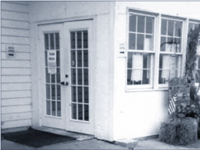
Image 15: Example of a voting location entryway made accessible by placing a wooden ramp over the entry threshold.
